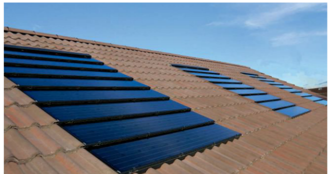
Advances in photovoltaic systems have made solar panels thinner, lighter and more efficient overall. Solar panels installed by European company Ecocetera mimic a traditional roof's layered configuration for a more seamless appearance.
