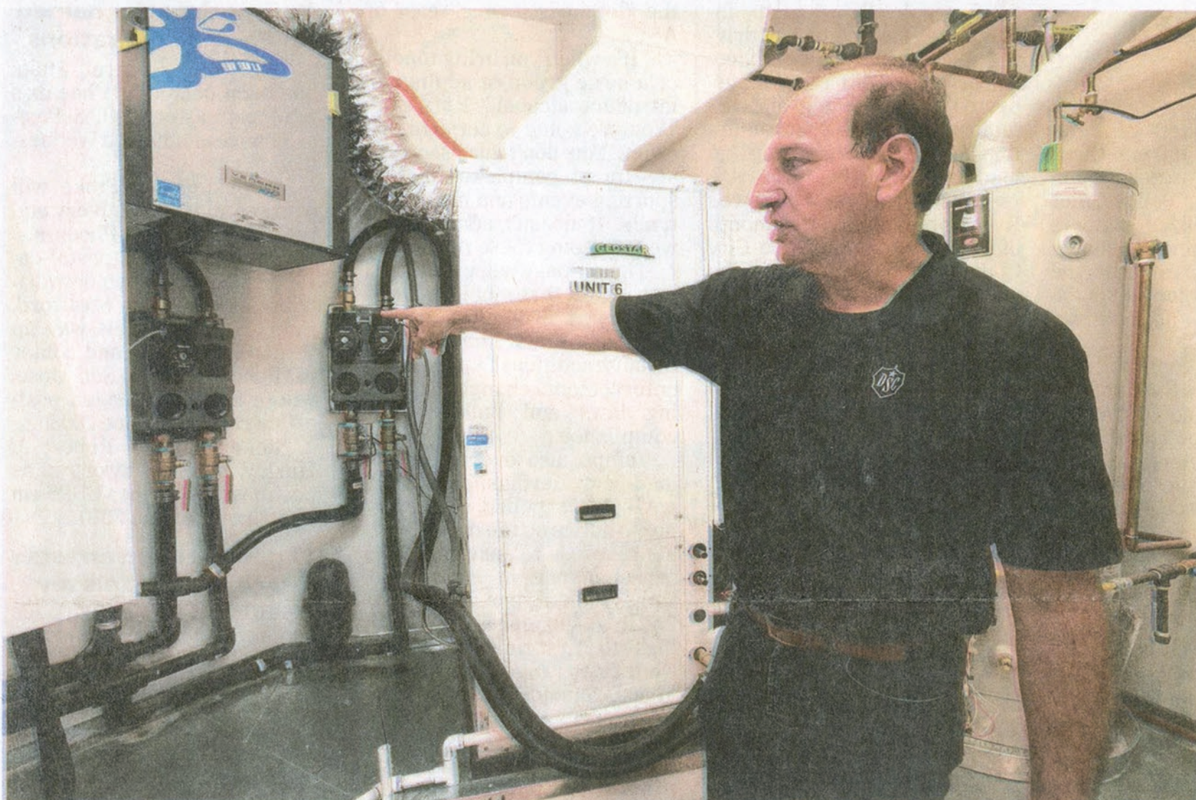
Jerry Meek, president of Desert Star Construction, points out parts of a geothermal heating and cooling system, which is installed in the first LEED-certified home in DC Ranch's Silverleaf community in Scottsdale. PHOTOS BY ROB SCHUMACHER/THE REPUBLIC
